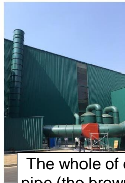
Spray in the exhaust pipe
