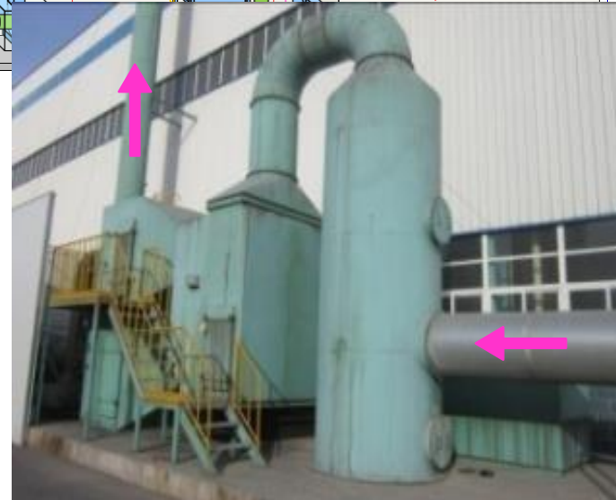
The whole of exhaust pipe (the brown area is the spray area)
